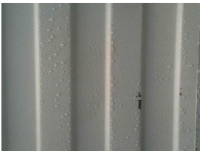
Moisture on container ceiling and walls due to inadequate ventilation
