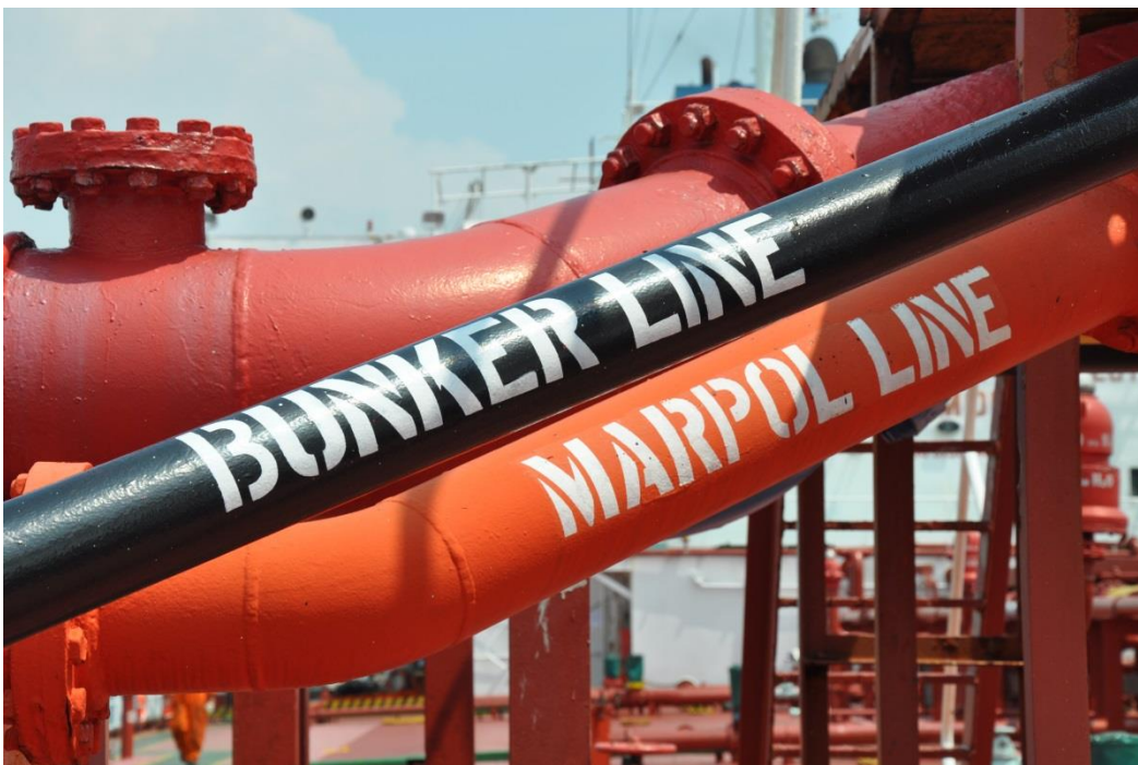
Bunker Fuel and Marpol Lines on a Tanker Vessel.
