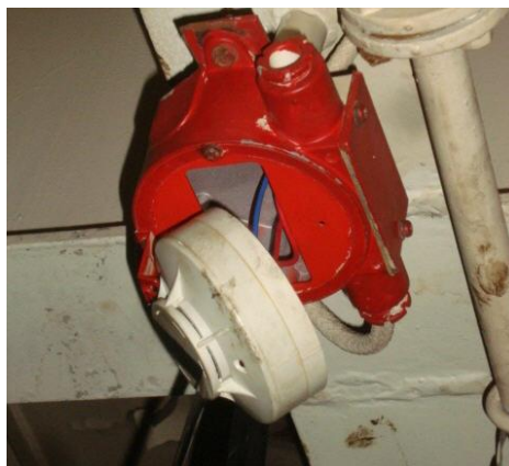
Fire detector above steering gear broken (Source: Skuld)
