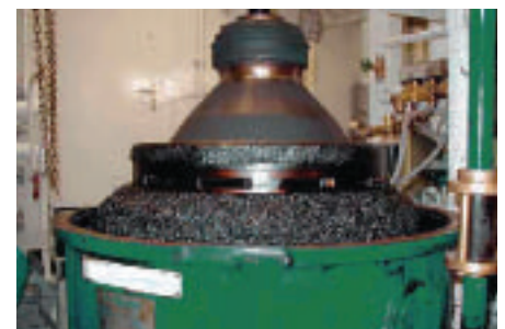
Excessive sludging in fuel oil separator
